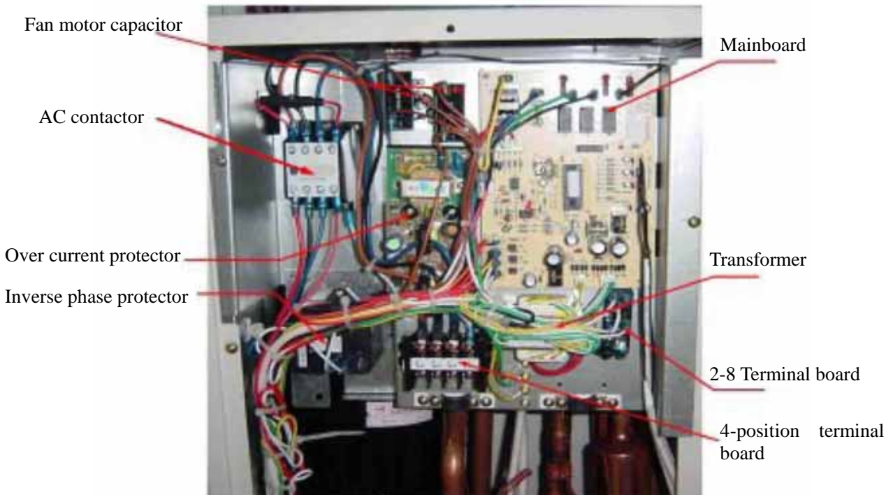
Outdoor unit electric box
