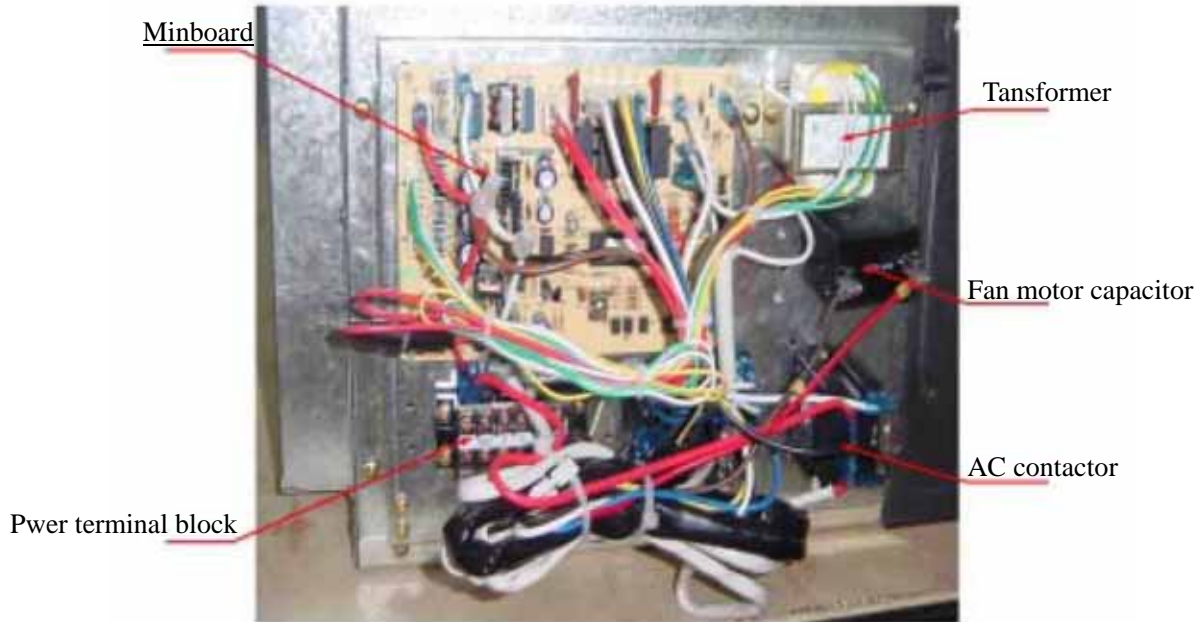
Indoor electric box
